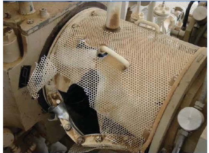
Fig. 21: VFD-induced Coupling Failure on 18000 HP LPG Compressor [15]
