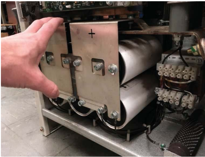
Fig. 16: DC Link Capacitors on 100 HP Inverter
